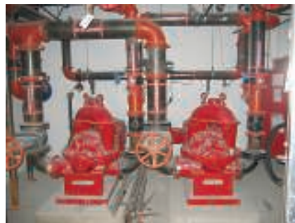
FIGURE 2. Shown here are several examples of fire-water pumps; an identical spare pump is commonly used to increase the reliability of fire-water pumping systems
