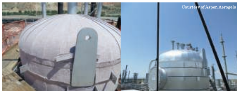
FIGURE 2. Localized insulation projects, such as the one shown here on the top head of a distillation column, are examples of engineered upgrades that can lead to improvements in energy efficiency
